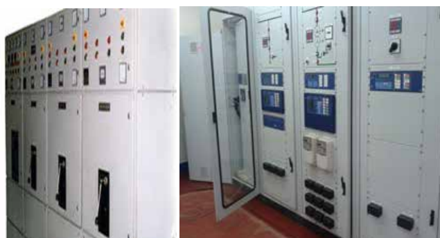
Protection and control bay Panels
