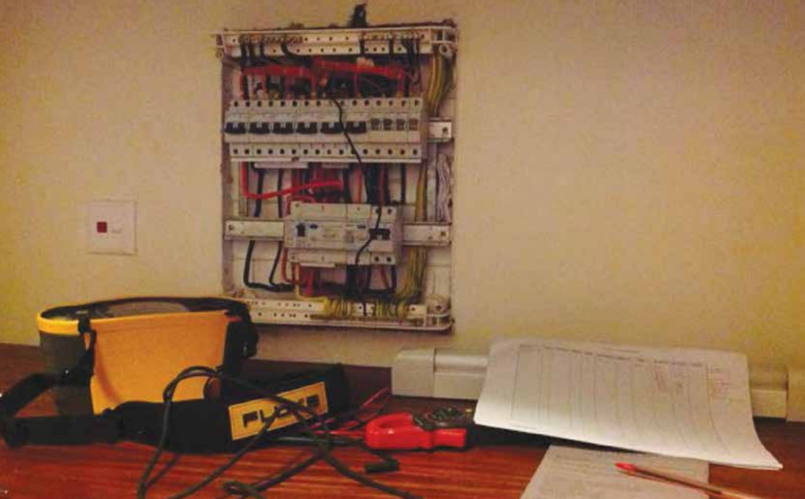
Carrying out a circuit protective conductor test after installation At a residential house.
